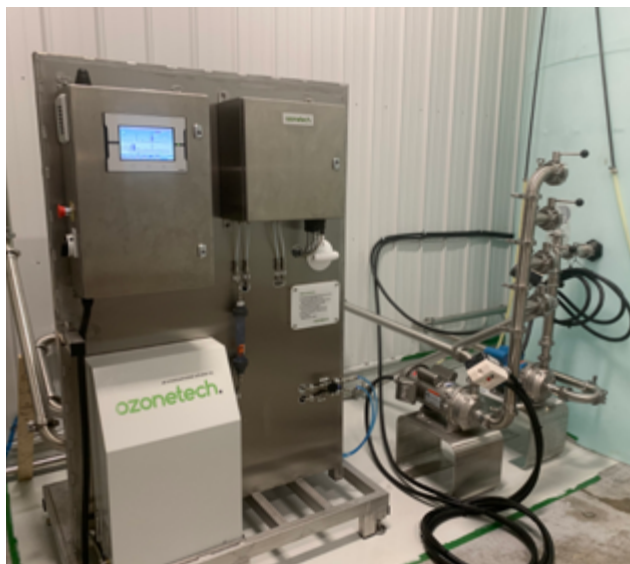
Ozonetech RENA Vivo A3 was installed easily thanks to the integrated connections, out-of-the-box automation and dissolved ozone control.
