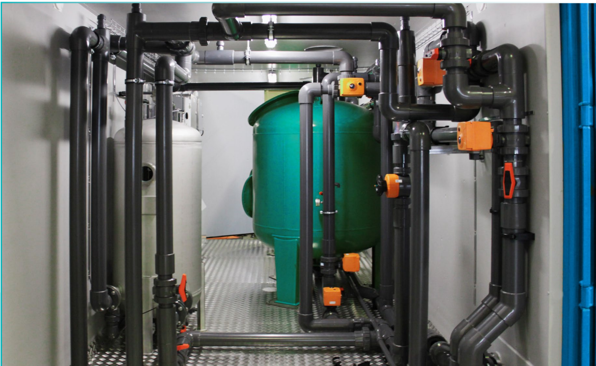
Internal view of the integrated filtration and ozonation system.
